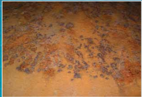
General corrosion on hull plate.
