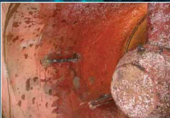
Corrosion around bow thruster.
