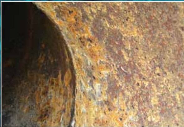
Pitting corrosion around exhaust discharge.
